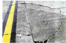
ABOVE Some of the predominant types of distress, which include structural cracking, surface cracking possibly owing to alkali-silica reaction (ASR), as well as pumping of fines and edge spalling
