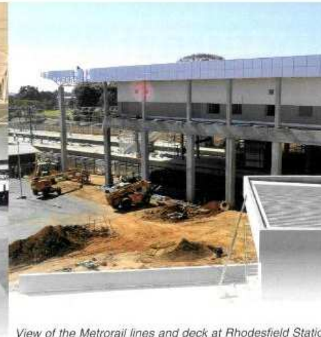
View of the Metrorail lines and deck at Rhodesfield Station seen from the Gautrain elevation
