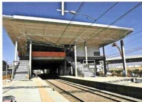
This view shows the relocated Metrorail tracks and newly constructed platforms, spanned by the commuter deck, with the elevated Gautrain line on the right
