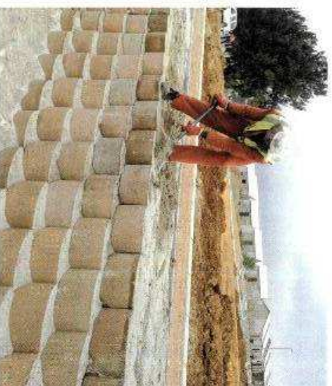
A Terraforce wall under construction, creating a level platform for roads and emergency housing in Kayamandi, near Stellenbosch.
