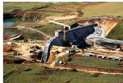
says Colin Logan, divisional manager: Dams, Hydropower and Underground Works at GIBB.
